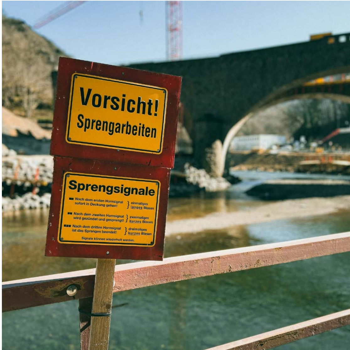
Sign reading "Warning! Blasting operations."
