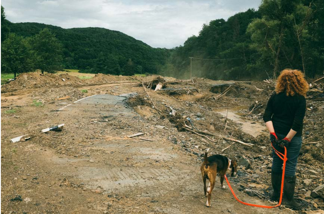
Surveying a section of road washed away by the Sahrbach.
